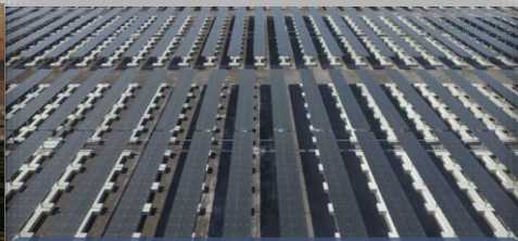
OSB Solar Park, Kayseri
